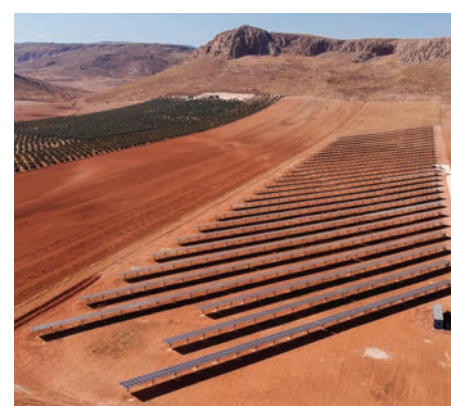
Solar PV plant in Namibia. © Villatonete / Shutterstock
